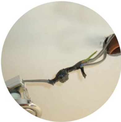
Unsatisfactory connections to a downlighter, requiring a Code C2
